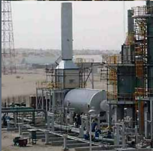
Top: Thermal Oxidizer and Hot Oil Heat Recovery, BHP Billiton/KBR Minerva Gas Plant.
