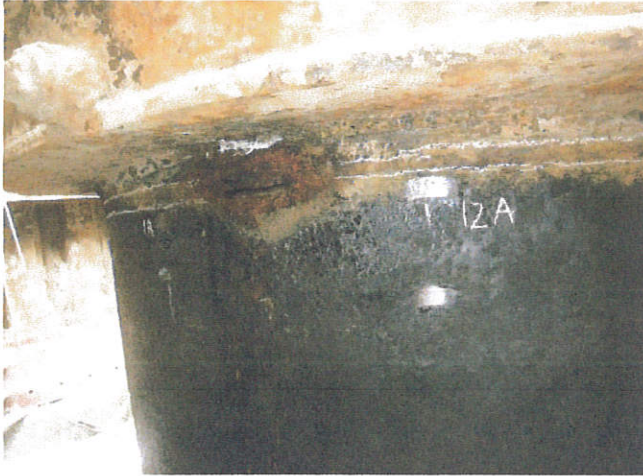
① Check the flaw at the connection part
