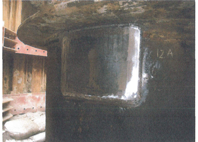
② First, weld the flaw with a iron plate. Then, apply Magicawrap-Steel to smooth the swelling.
