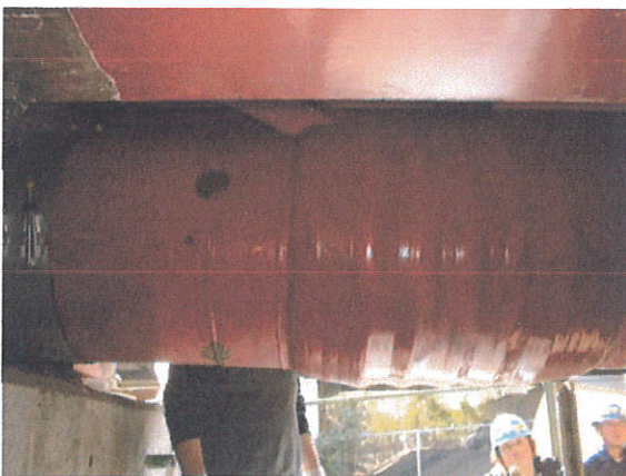
⑨ Corrosion is found in several spots on the straight portion
