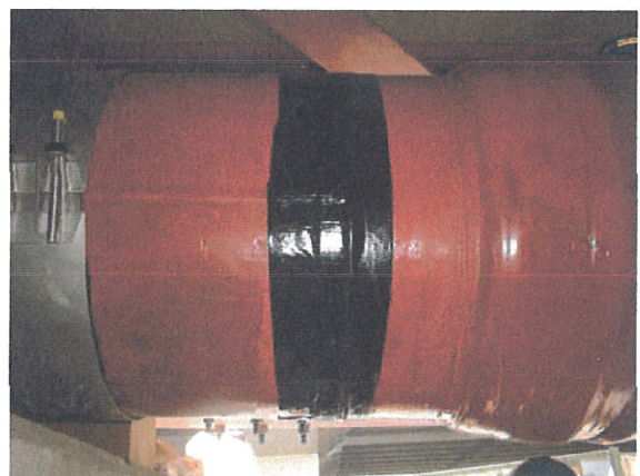
⑩ First, wrap the Butyl roll as pre-treatment of the Magicawrap. Then, wrap the Magicawrap to squeeze 1-2 minutes to finish
