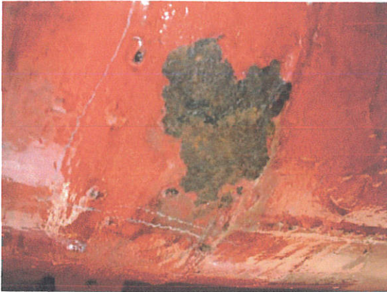
⑥ water is running on 1 spot due to the corrosion
