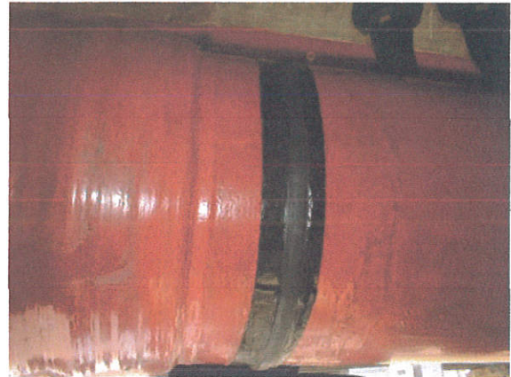
⑦ On the spot, wrap the Butyl roll, and then Magicawrap-tape to stop leak
